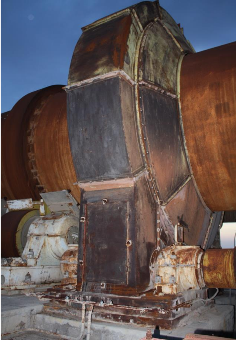
15c) The main drive of the furnace
