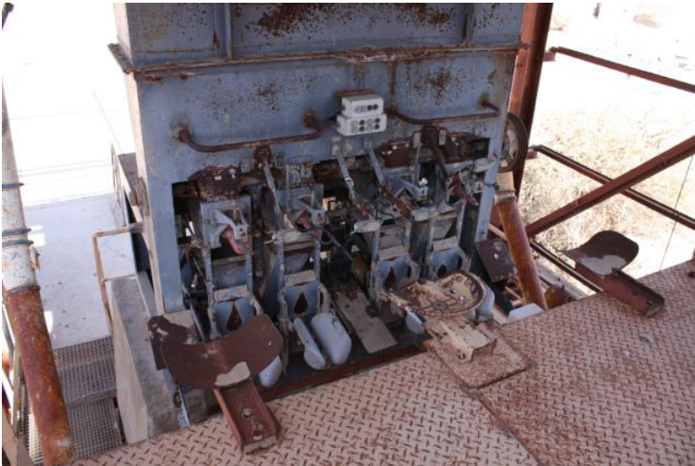
34d) Cement filling machine
