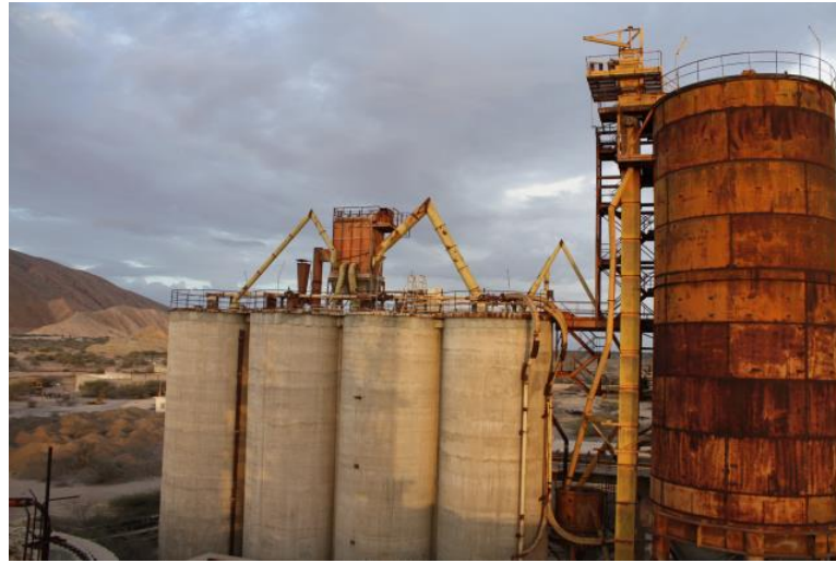
11a) Homogenization storage
