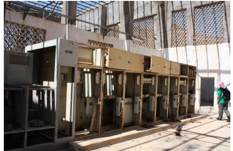
60) Substation energy 6 kW
