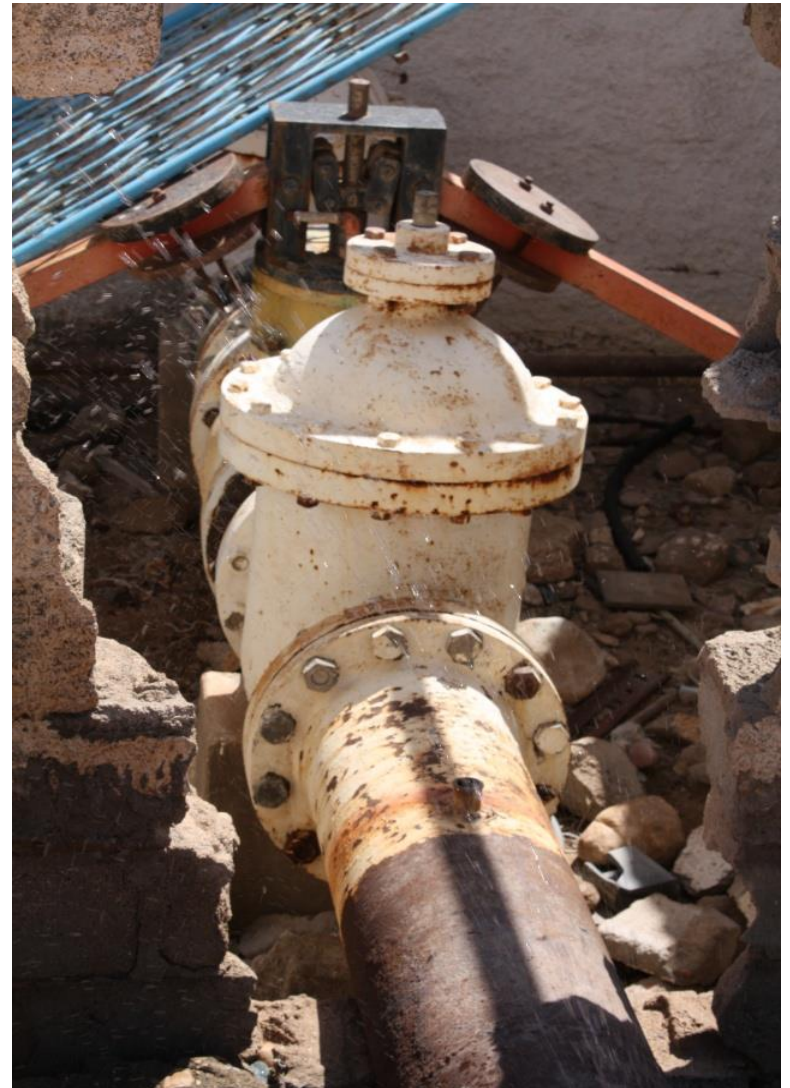
85) The main water valve
